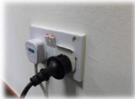
Use of not permitted plugs
